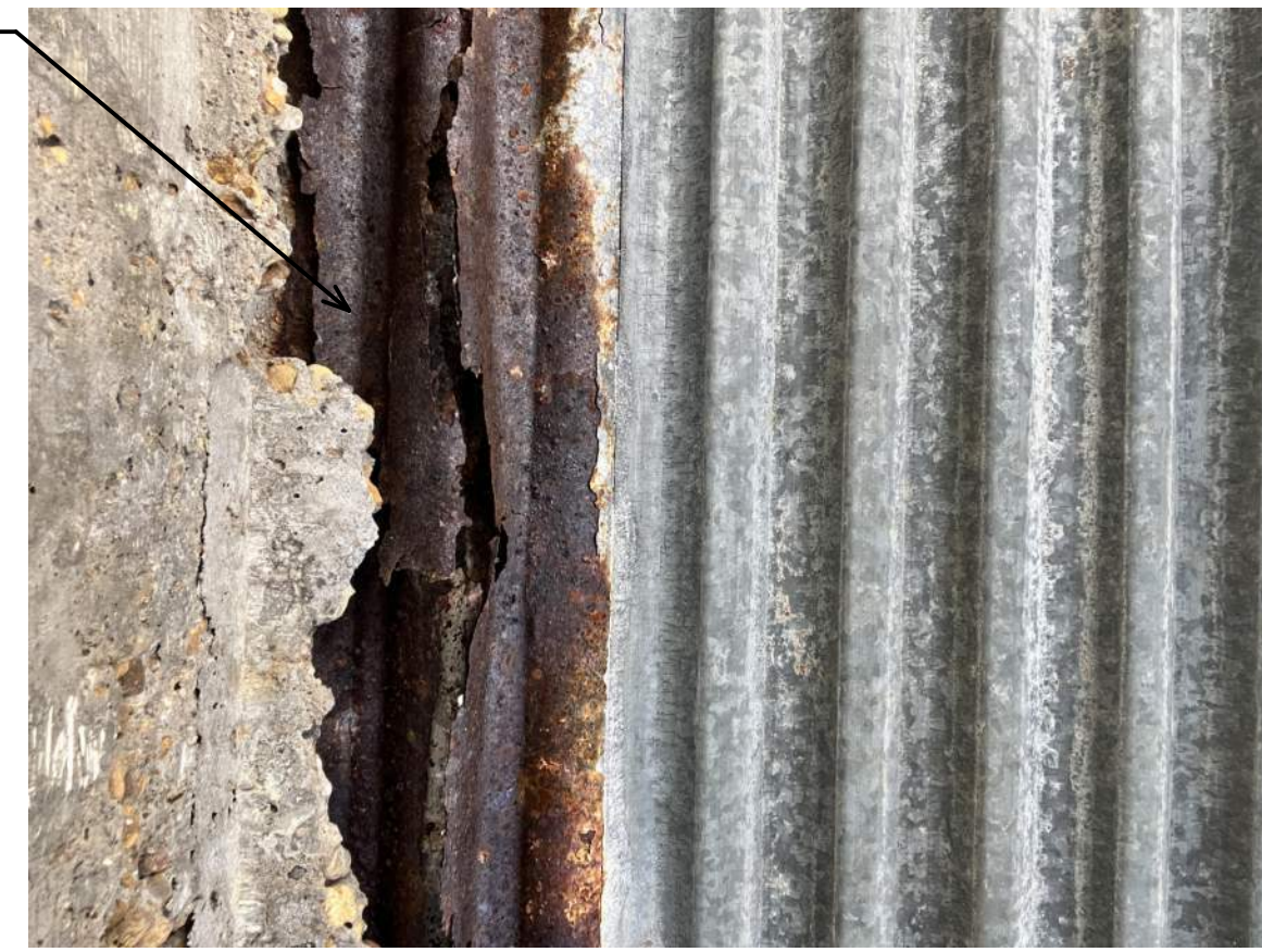
6 DETERIORATED BRIDGE DECKING NO SCALE
